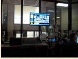
Control Room, Lincoln County Jail, Hugo, Colorado
